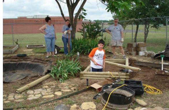
Cleanout nearly finished and new bog is under construction with the willing help of a 4 th grade student, 2 pond society members, and several teachers.
