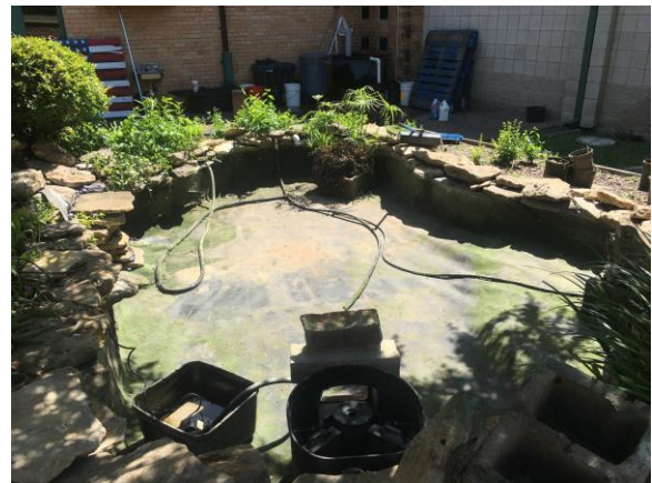
Skimmer and bog pump box
